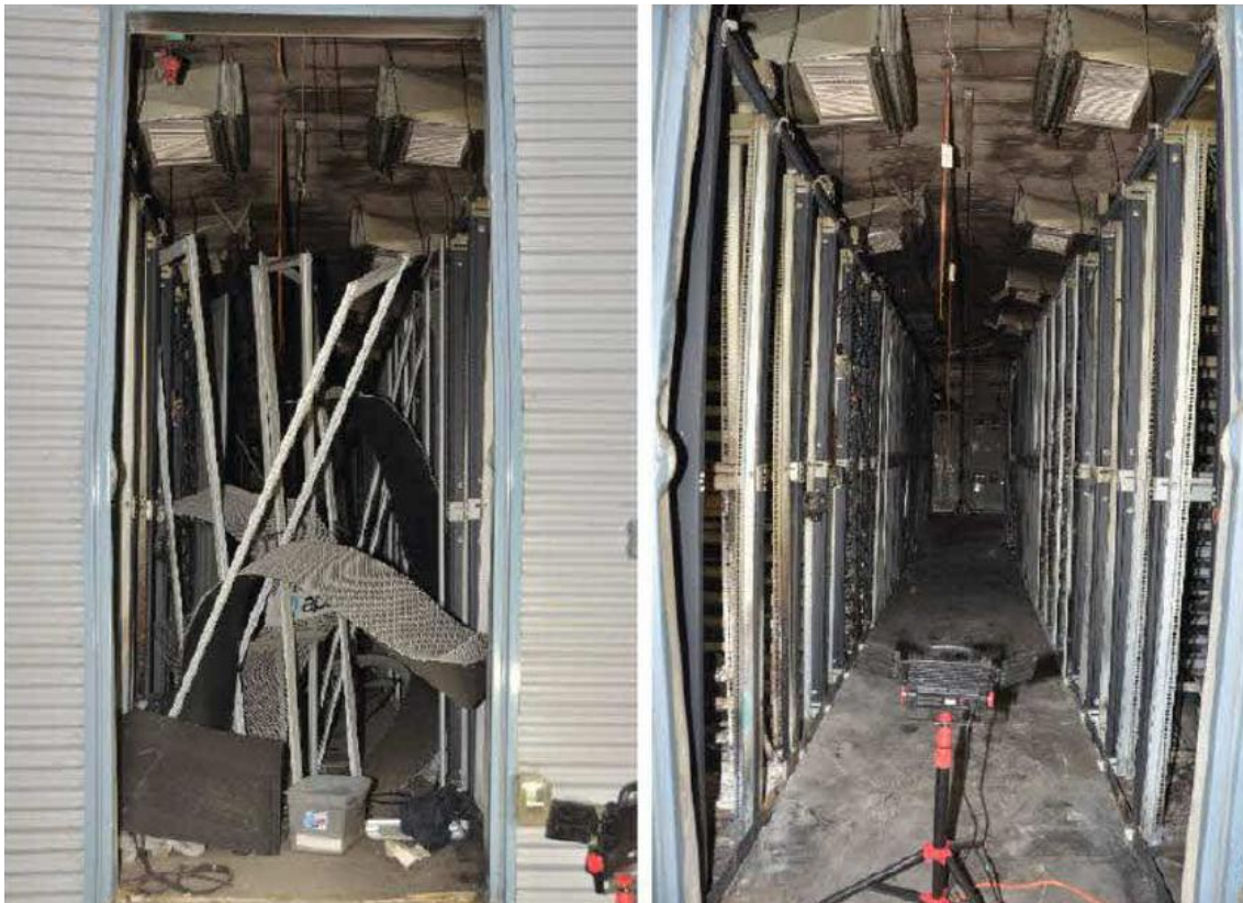
Figure 4 – BESS contained post deflagration event 7
