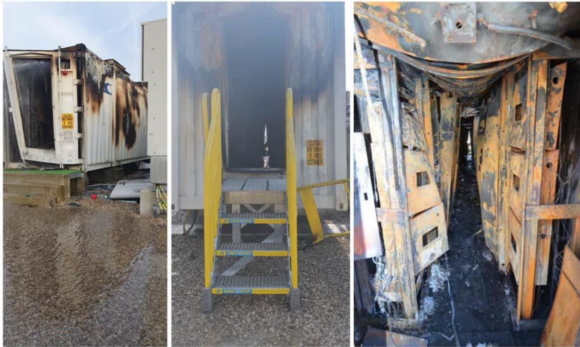
Figure 7 – Post incident photographs 12
