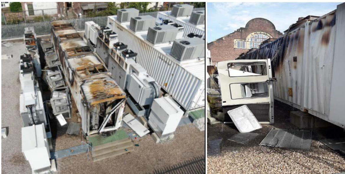
Figure 6 – Post incident photographs 11
